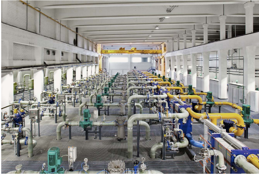
Fig. 3: Grey Space, Google Data Center, Cooling Plant, Hamina, Finland. Source: https://www.google.com/intl/de/about/datacenters/gallery/#hamina-cooling-plant , protected by copyright
